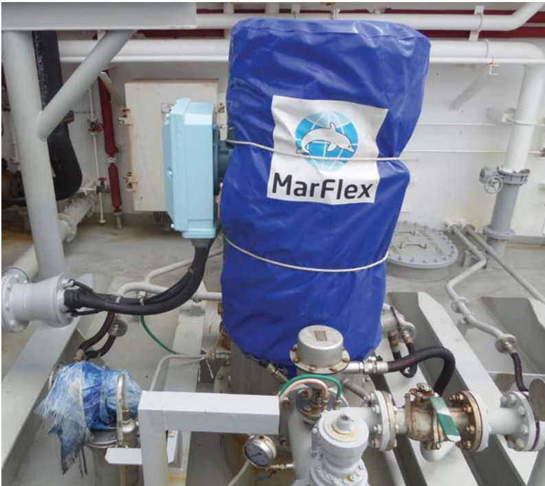
Marflex Variable Frequency Drive Cargo pump.
